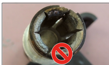
Fig. 14: Socket contact contaminated due to acid exposure
